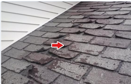
1.0 Item 1 (Picture) Damaged/lifted shingles with granule loss need to be evaluated/repared by a licensed roofing contractor
